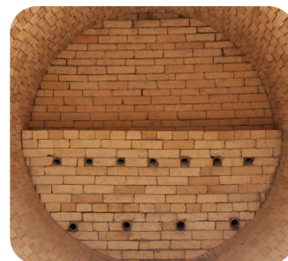
Figure 4: Drying oven lined with refractory bricks
