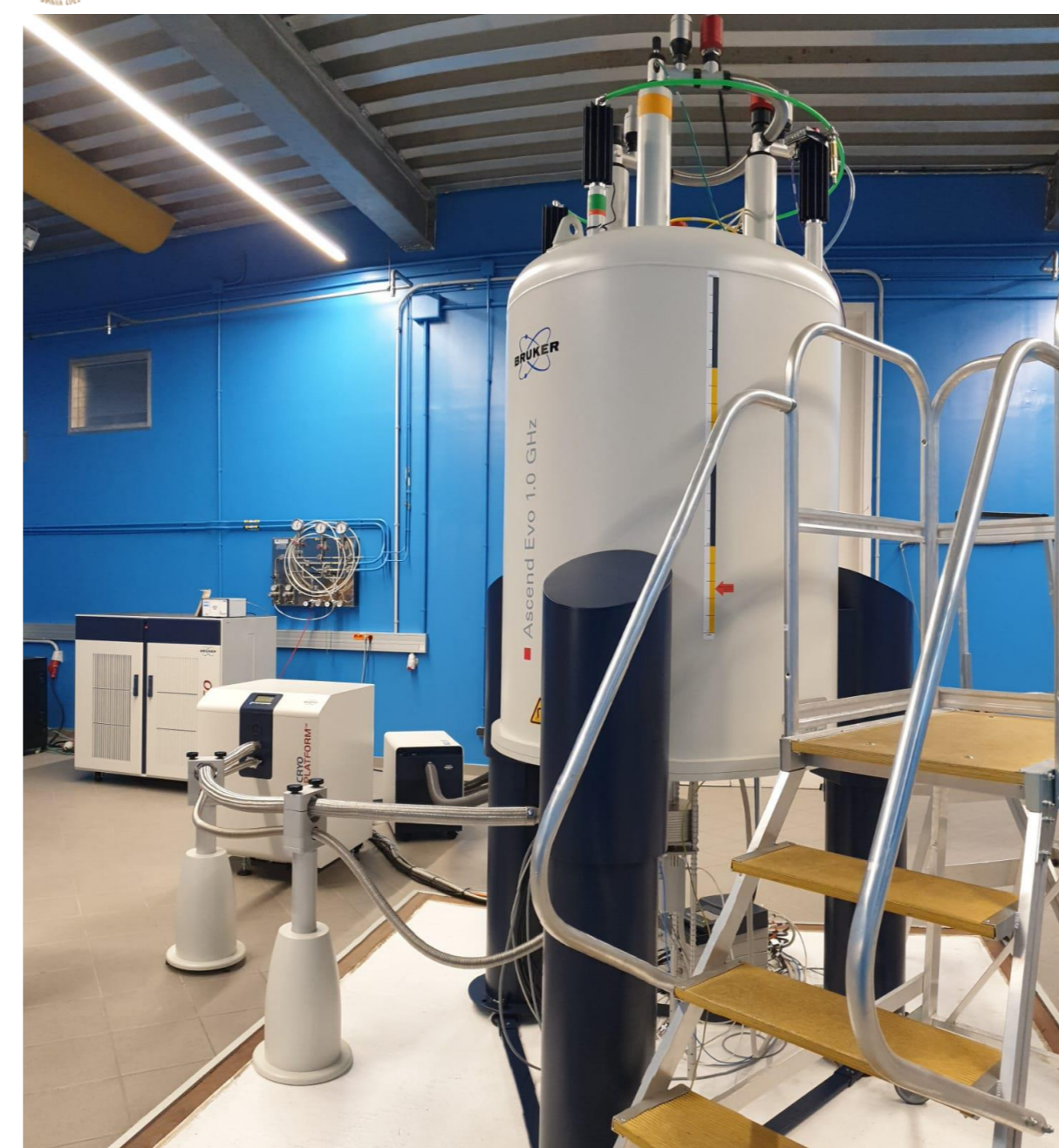
The Ascend Evo 1.0 GHz installed at the University of Barcelona for the BioNMR Group led by Prof. Miquel Pons Valles.
