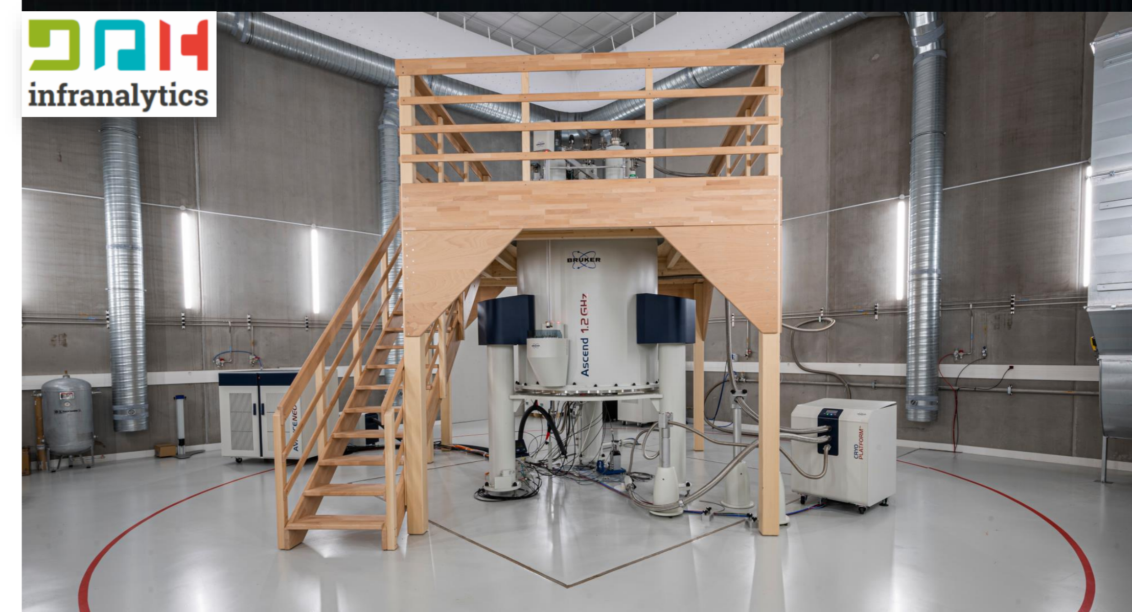
The Ascend 1.2 GHz installed for CNRS - Infranalytics at University of Lille, France, Courtesy of Prof. Olivier Lafon.
