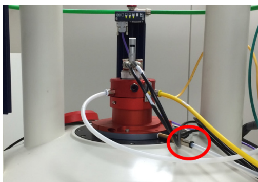
Figure 6: Shim cooling piping to magnet
